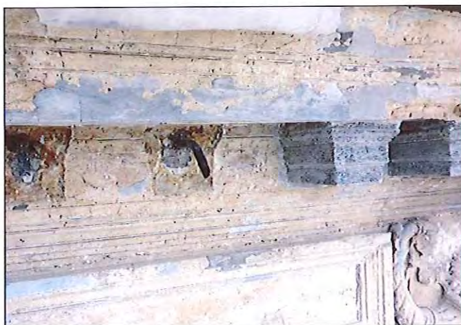
Photo fer corrodé
